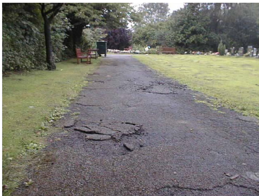
Carnforth Cemetery – a path in need of repair
